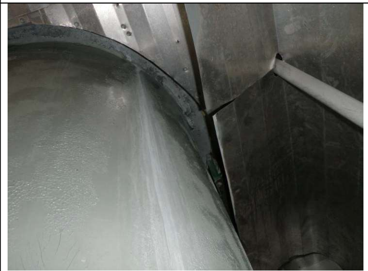
Roof Seal leaking
