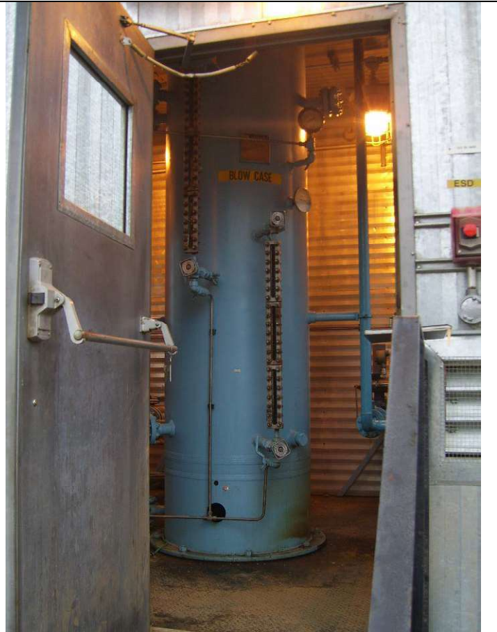
Vessel External Over View
