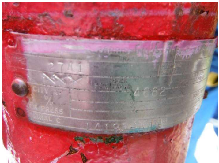
PSV data plate – 2006 service tag is not attached.
