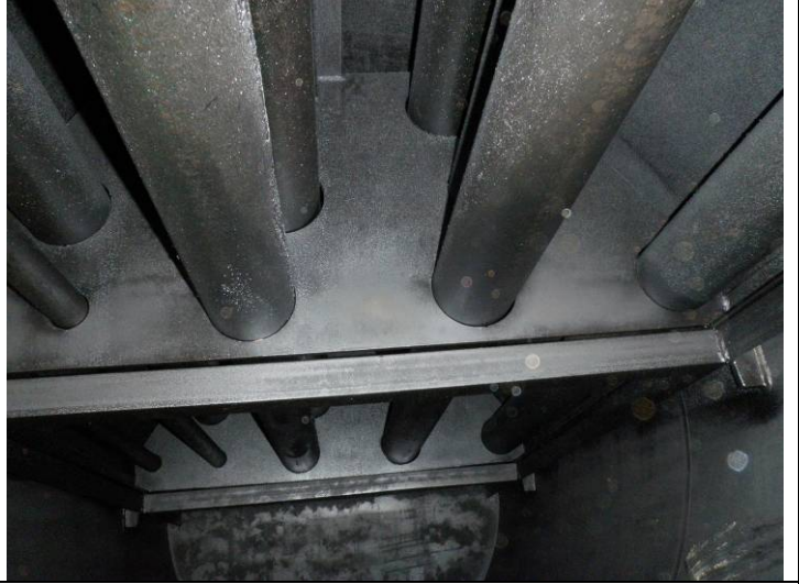
Piping and Support Channels
