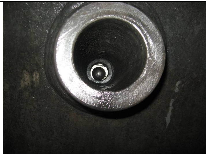
High level control
