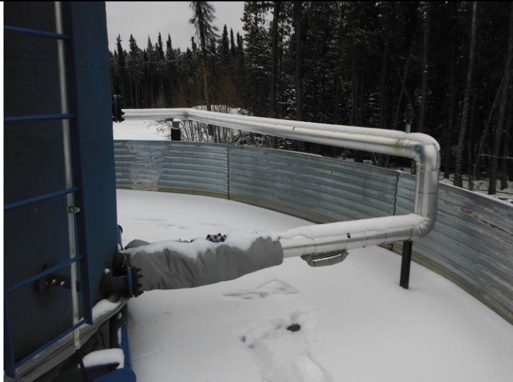
Valves and piping well supported
