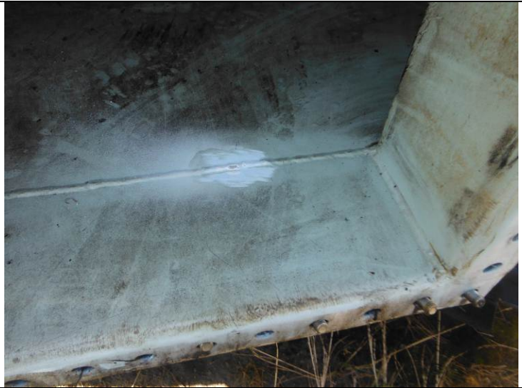
Coating chip repaired at time of inspection
