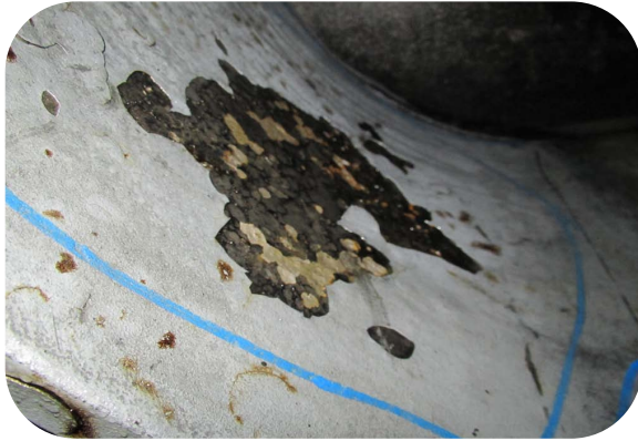
A2710237_Close up of the nozzle pitting_10Oct2012
