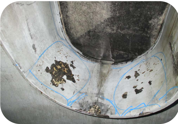
A2710237_Sealed manway nozzle pitting_10Oct2012
