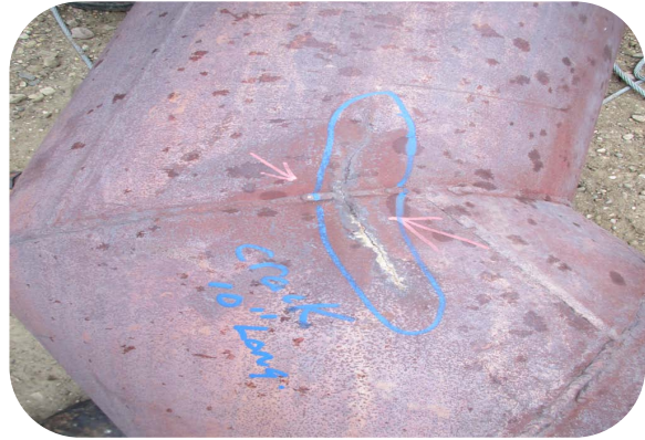
A2710237_10" Crack identified_10Oct2012
