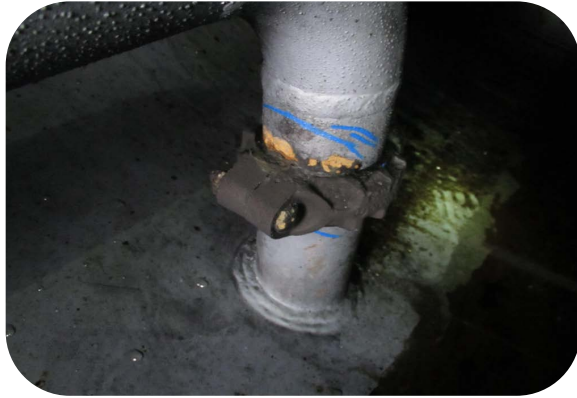
A2710237_Severe corrosion of the vic clamp_10Oct2012
