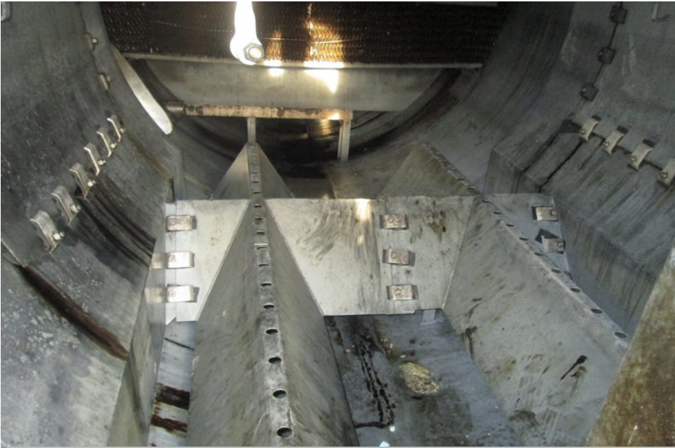
V-shrouds below firetubes are in good condition.
