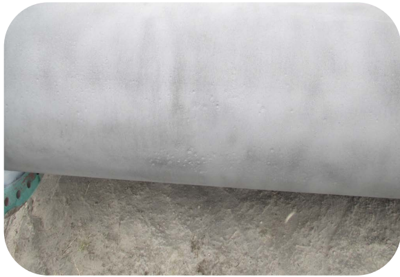
A2710237_External pitting 0.030" on tube legs_9Sept2014
