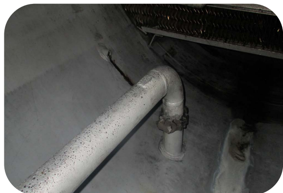
A2710237_Internal piping secure_9Sept2014
