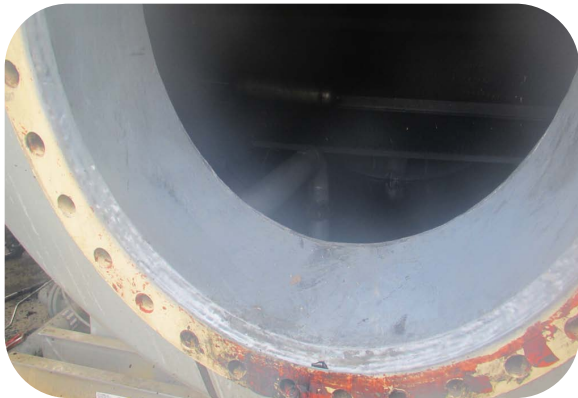
A2710237_West head manway nozzle_9Sept2014
