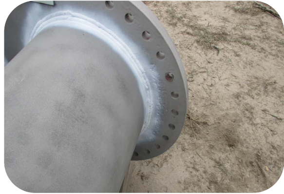
A2710237_Tube sheet corrosion 0.060" deep 1" wide 20" long_9Sept2014
