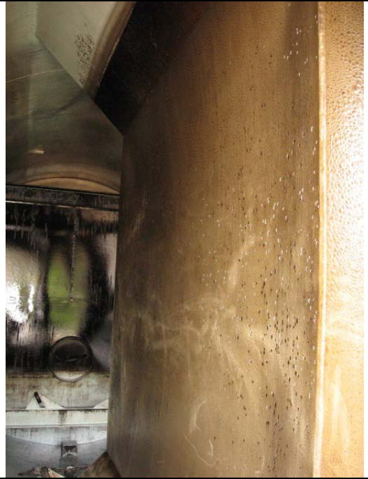
Inlet chute – deformation and blistered coating.
