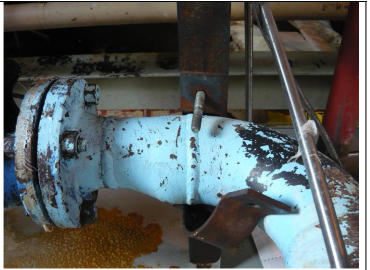
Loose support clamp
