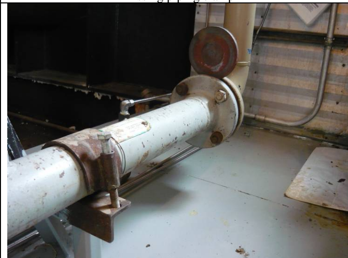
Loose Piping Clamp
