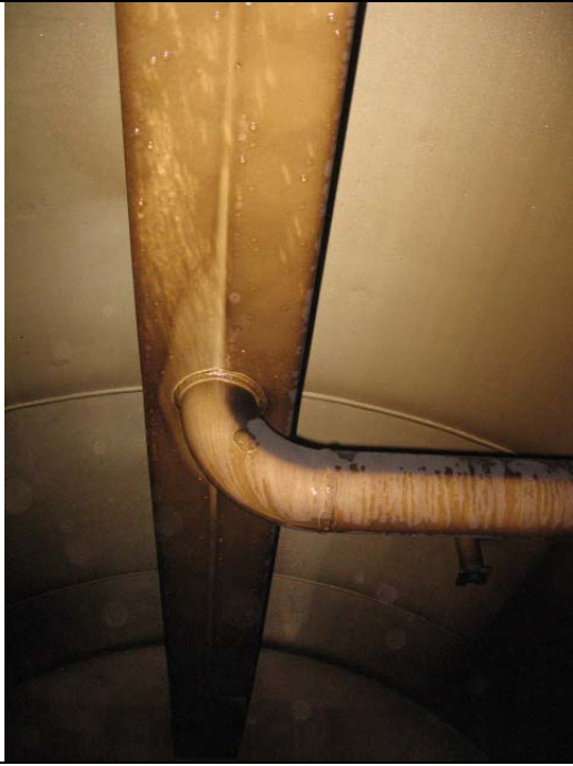
Oil outlet piping in top section of Treater
