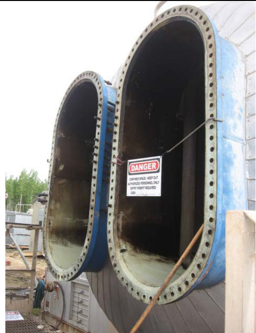
Fire tube access areas
