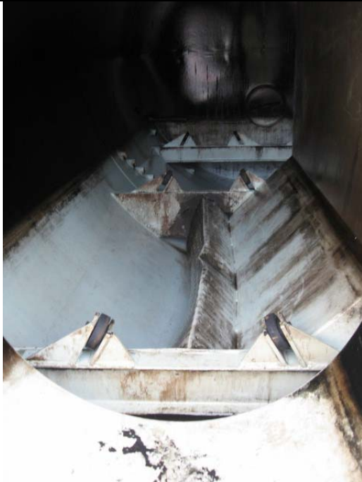
Opposite side – sparging chute in front end – notice deformation.
