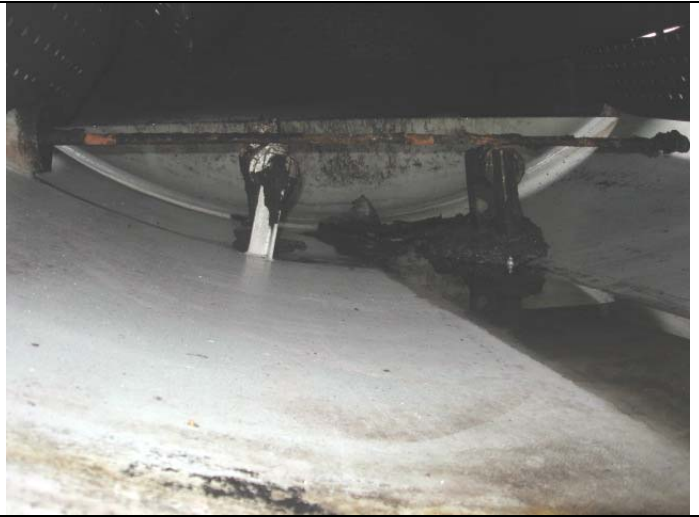
Anode in front end – completely consumed
