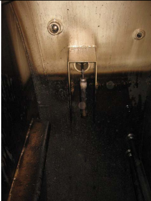
Oil level control in between weirs
