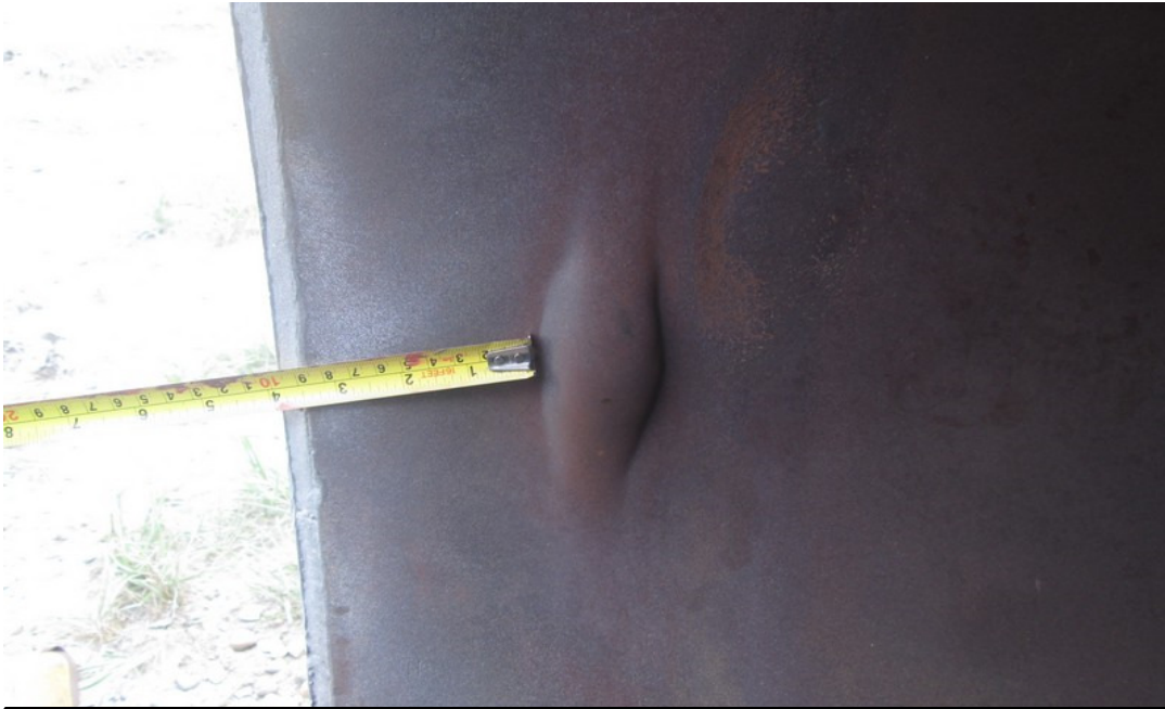
Firetube bulge/blilster on internal diameter of firetube (coldside) at same position as tubesheet. Height of bulge/blister is about 15 mm above parent metal, thickness of tube is 12.6 mm.
