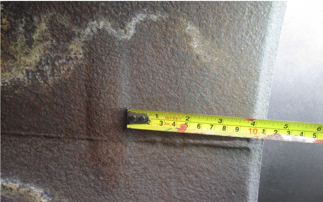
Firetube bulge/blilster on internal diameter of firetube (coldside) at same position as tubesheet. Height of bulge/blister is about 4 mm above parent metal, thickness of tube is 12.6 mm.
