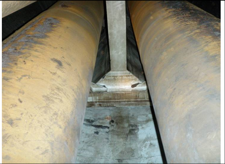
Lower shell and fire tubes
