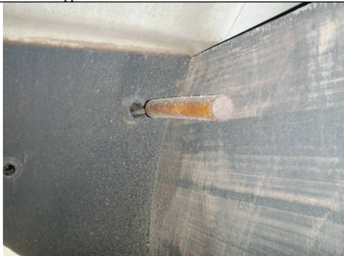
Oil level float and weir
