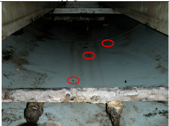
Anodes - 30% loss - coating failures
