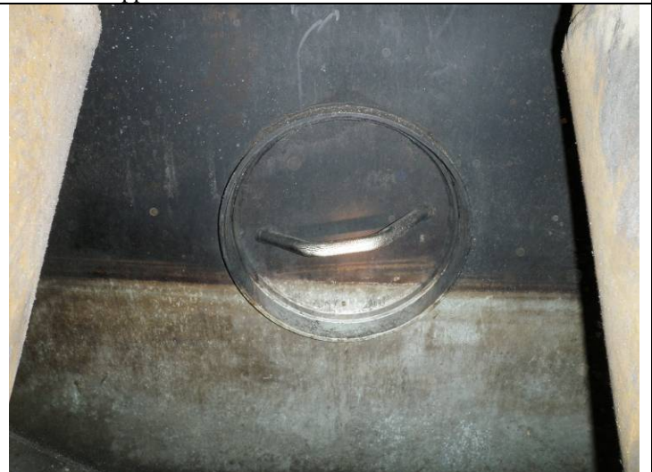
Internal weir manway
