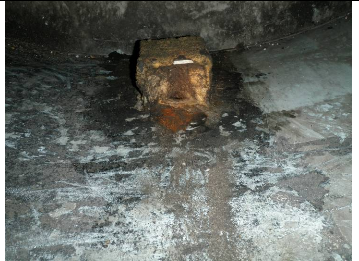
Oil drain/vortex – calcium buildup – flow restricted
