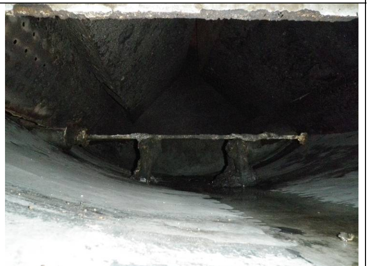
Anode - 100% loss (looking towards Fire Tube end)
