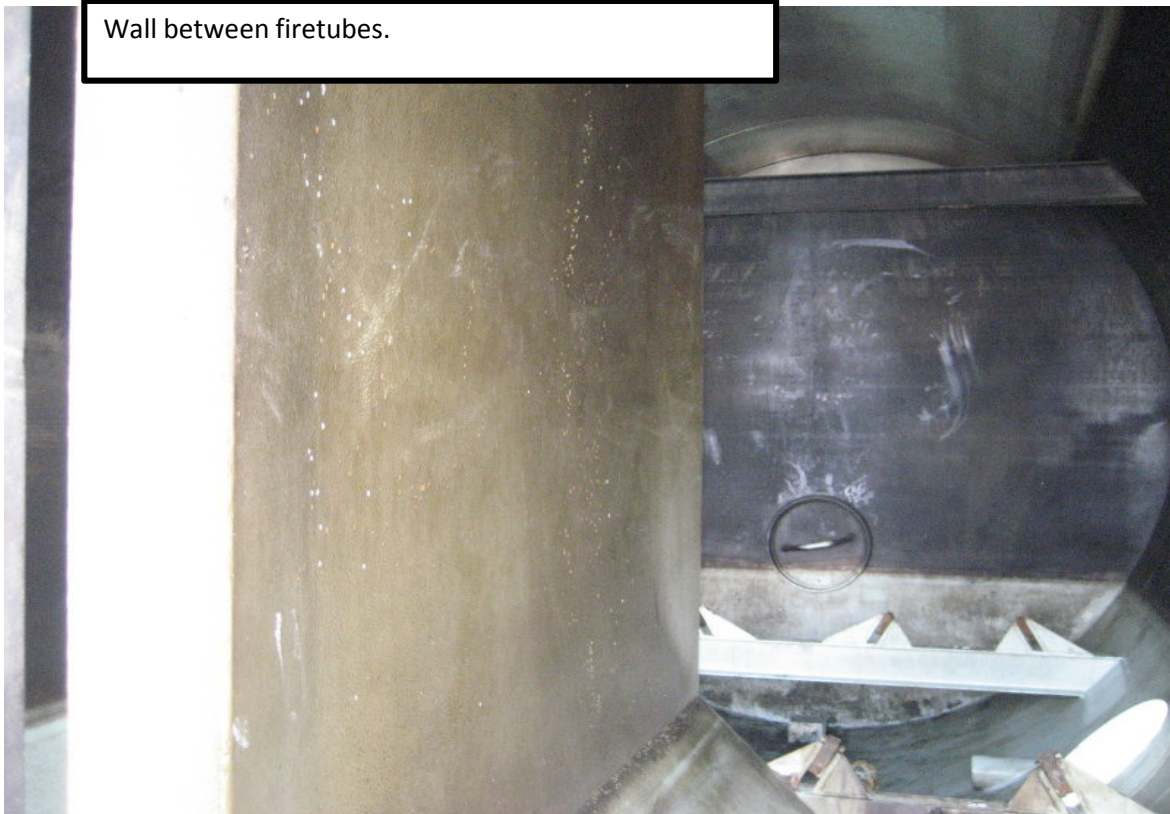
Nozzles after scale had been chipped away.
