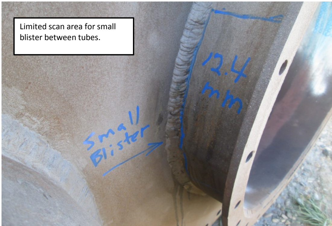
Limited scan area for small blister due to gusset. Firetube not turned over for inspection.
