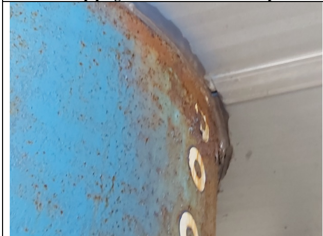
Surface corrosion below roof
