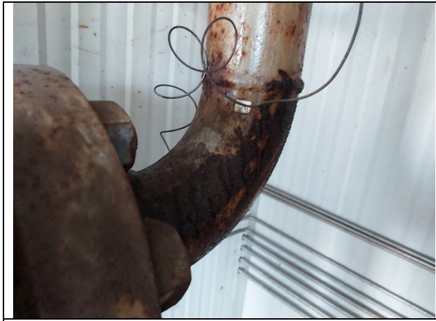
Outlet piping – surface corrosion – no pits
