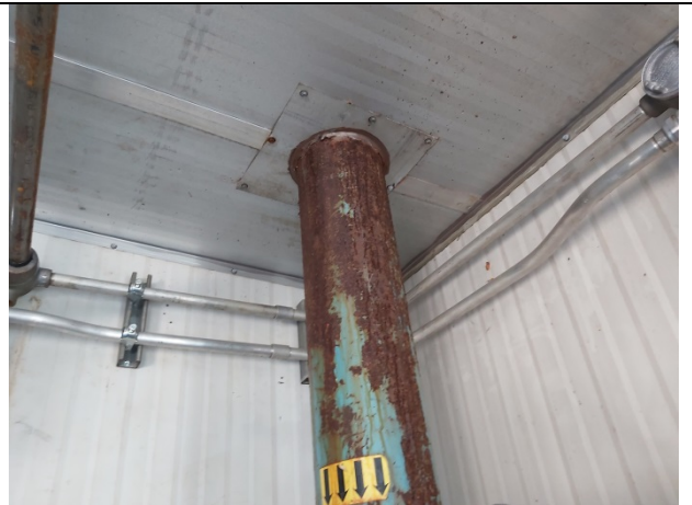
Outlet piping – surface corrosion
