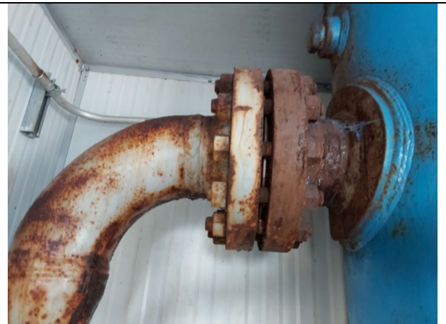
Inlet – surface corrosion present – no pits
