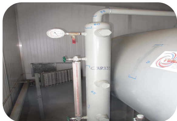
C38332_6" Bridle intact secure and Liquid level sight glass intact_18March2013
