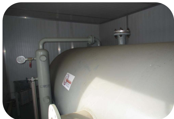
C38332_Top Shell and Bridle associated piping_18March2013
