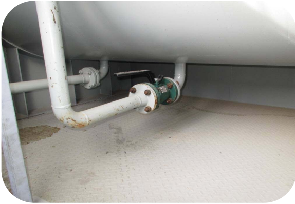
C38332_Bottom 2" Outlet Piping intact_18March2013
