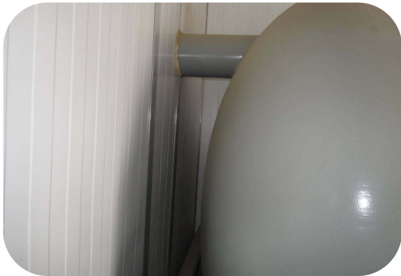
C38332_South End 6"Outlet Nozzle and south head_18March2013
