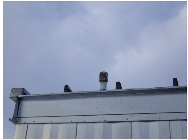
PSV INLET PIPING (NO PSV)
