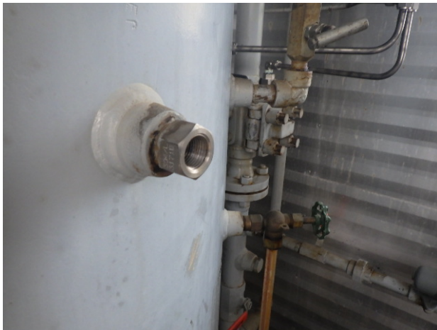
MISSING PLUG ON THREADED CONNECTION (SHELL)
