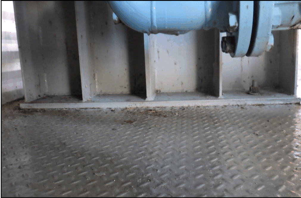
ANCHOR BOLTING MISSING
