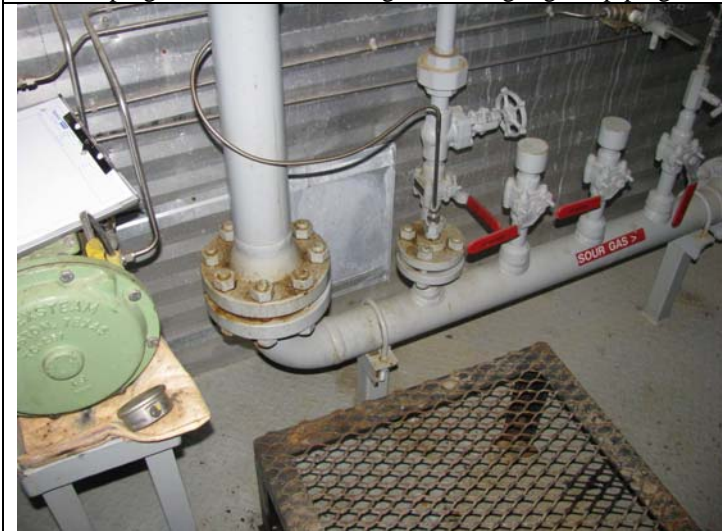
Outlet piping is in good condition and well supported.
