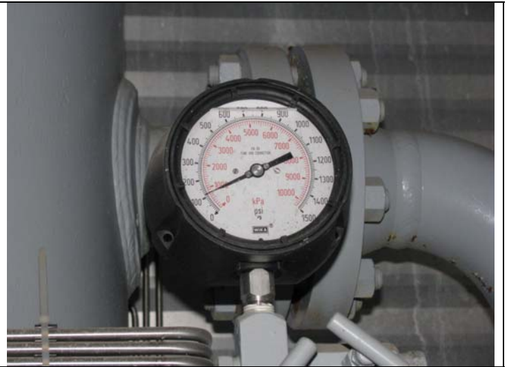
Gauges are in good condition and within range for the MAWP.
