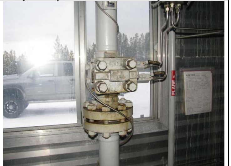
Choke is in good condition with no leaks.
