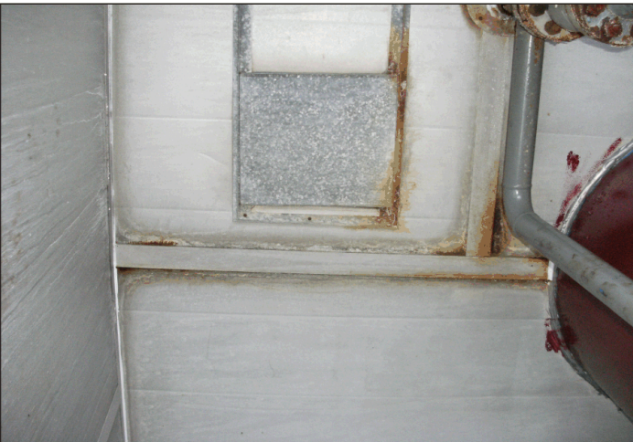
DETERIORATION ON BUILDINGS ROOF
