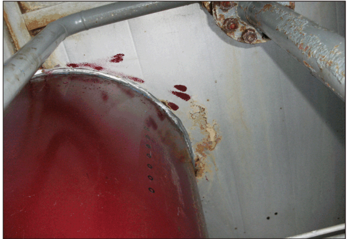
DETERIORATION ON BUILDINGS ROOF
