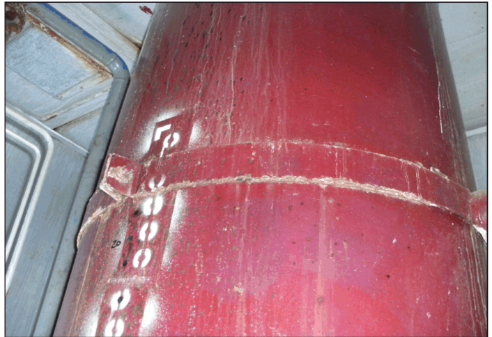
PAINT FLAKING AND RUSTING ON SHELL
