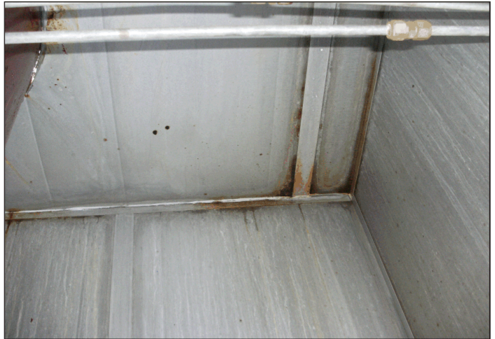
DETERIORATION ON BUILDINGS ROOF
