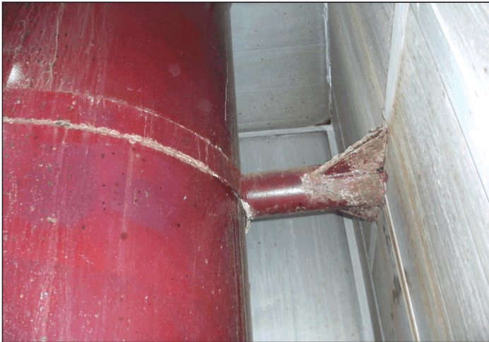
PAINT FLAKING AND RUSTING ON SHELL
