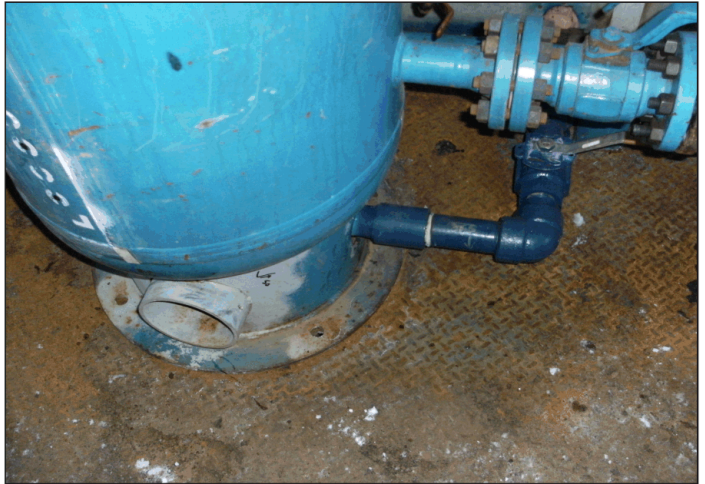
THREADED DRAIN PIPING
