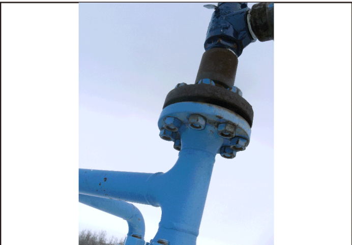
FLANGE BEFORE PSV INLET IS SHORT BOLTED
