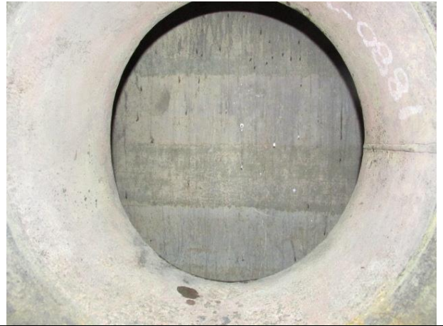
Baffle plate across from manway, limits internal cleaning and visual to half of vessel only
