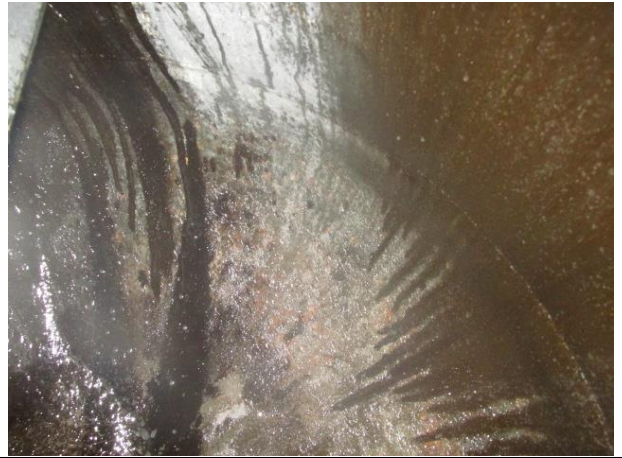
Bottom shell to head weld
