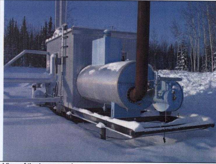
View of the burner end
