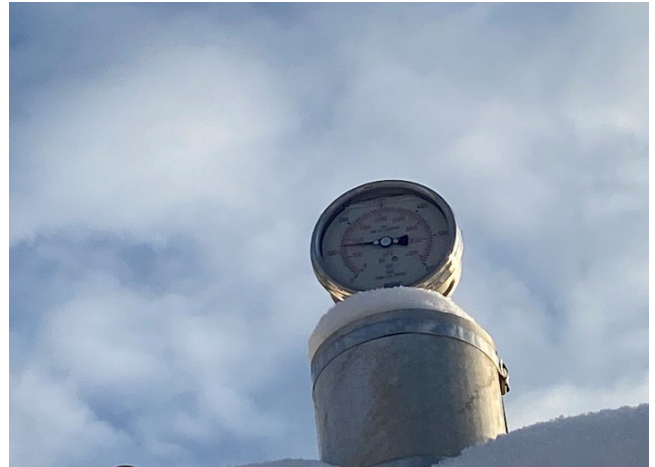
Picture 10: Pressure Gauge
