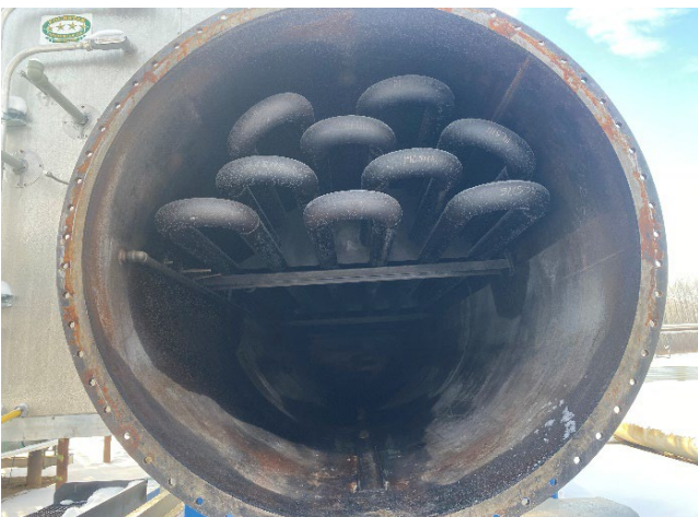
Picture 11: Internal Vessel Overall
