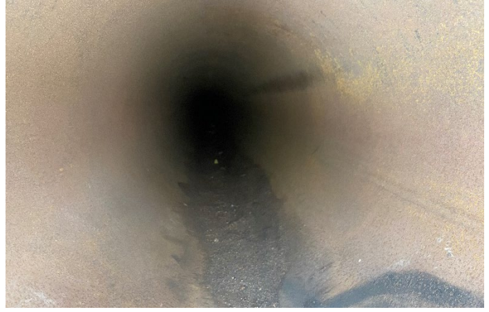
Picture 6: Internal Tube Overall
