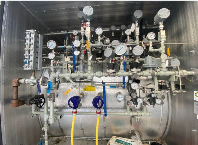
Picture 9: Piping, valves and gauges
