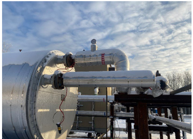
Picture 4: Flanges still partially connected
