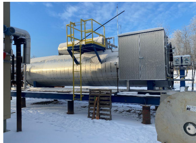
Picture 6: Vessel Overall
