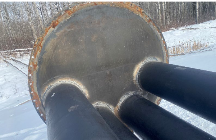
Picture 3: Internal Tube Sheet Flange
