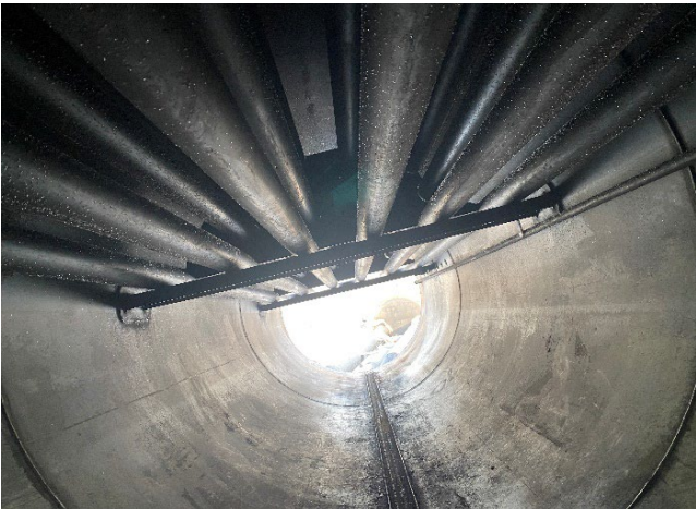
Picture 15: Internal vessel overall
