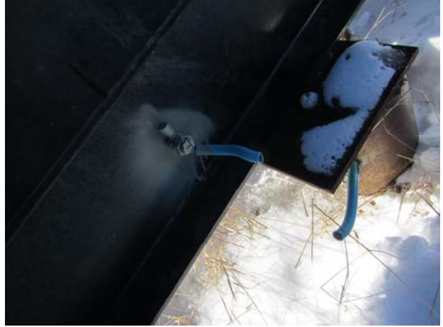
Ground Cables Cut
