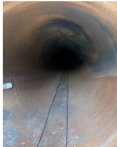
BURNER SIDE INTERNAL OVERVIEW
