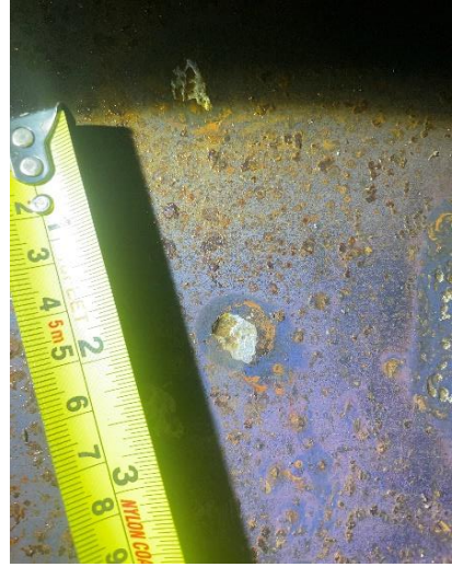
TYPICAL CORROSION CLOSE UP AT BACK END
