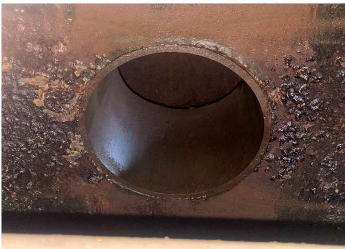
EXPANSION TANK NOZZLE
