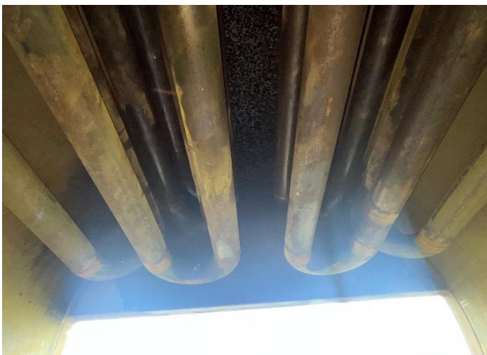
FRONT END RETURN BENDS OVERVIEW
