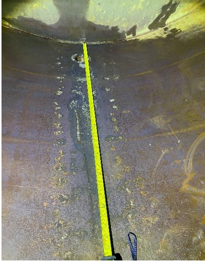
GENERAL CORROSION AT BACK END OVERVIEW
