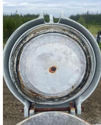
EXPANSION TANK THIEF HATCH GASKET CONDITION
