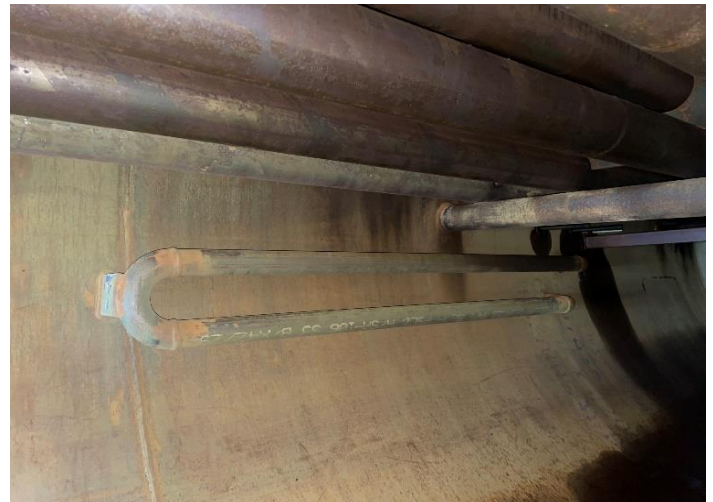
FUEL GAS COIL PIPING
