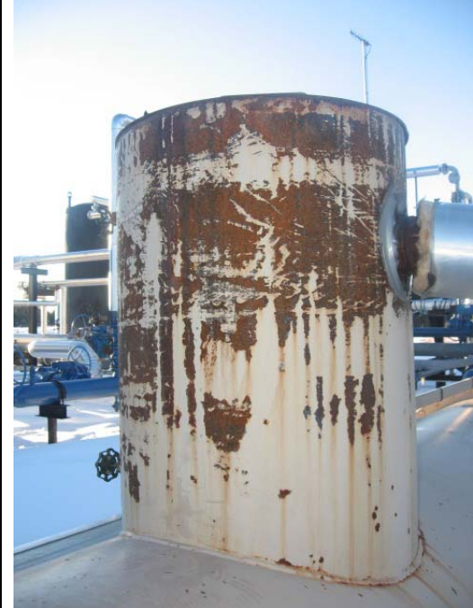
Accumulator – missing paint
