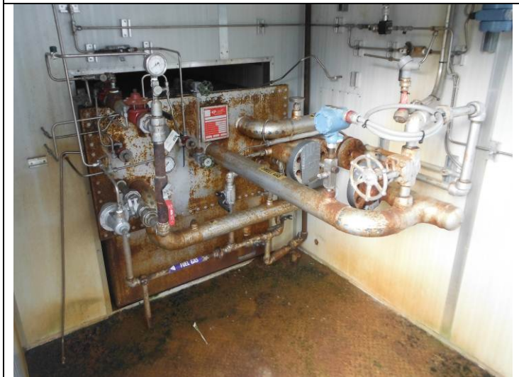
Line heater removed from service
