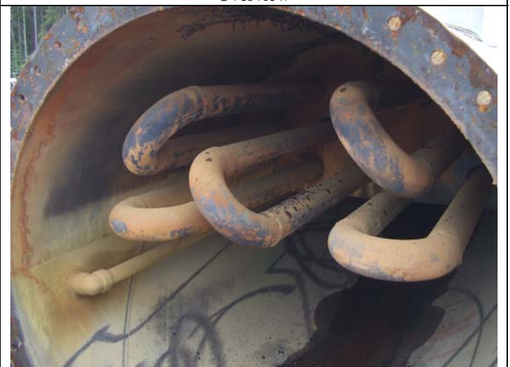
Heater coil overview
