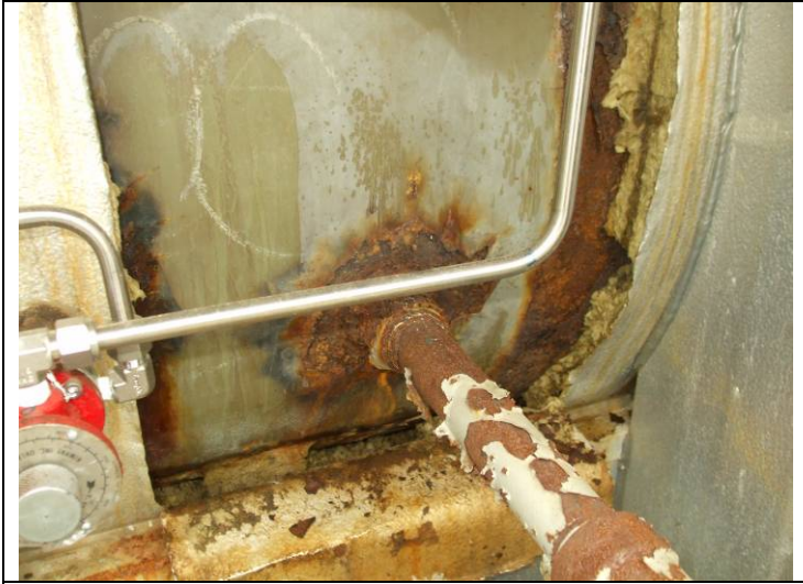
Shell external corrosion
