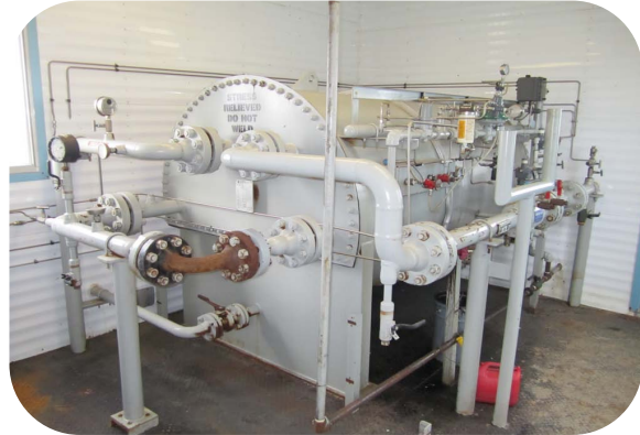
A0438939_Inlet and Outlet piping_28Mar2012
