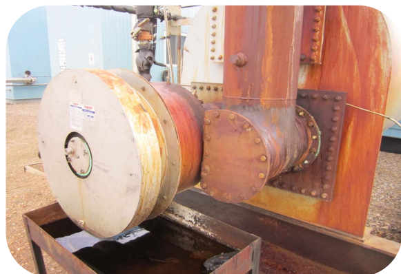
A0438939_Burner and Stack assembly_28Mar2012
