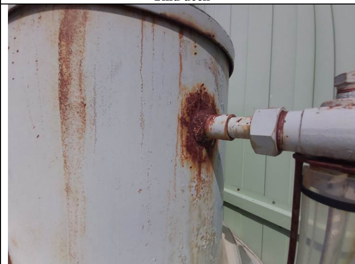
Surface corrosion on accumulator / expansion tank
