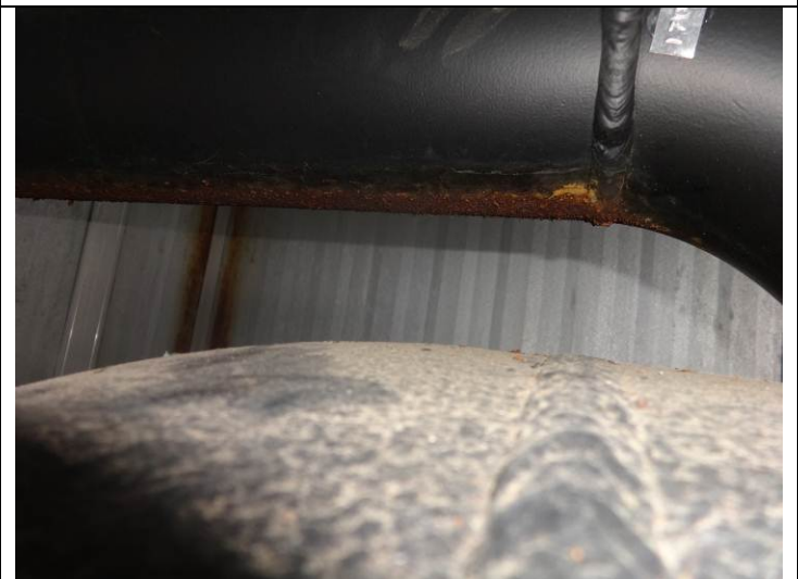
Corrosion on piping
