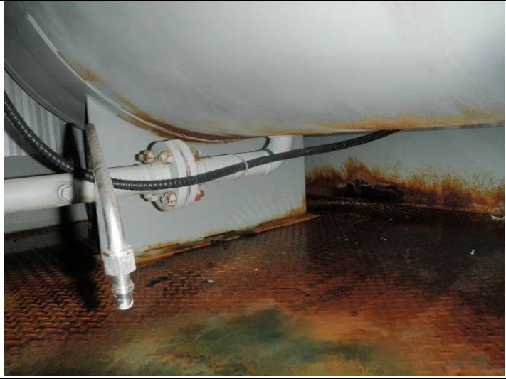
Standing water - Surface corrosion
