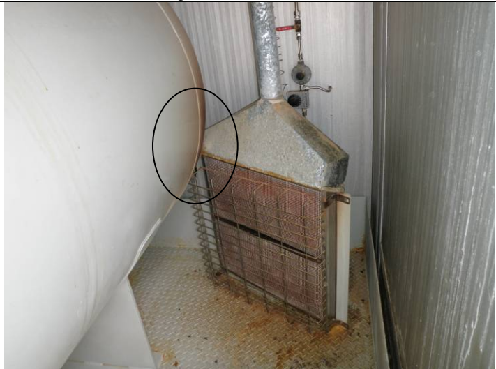
Catadyne Heater – close proximity to vessel
