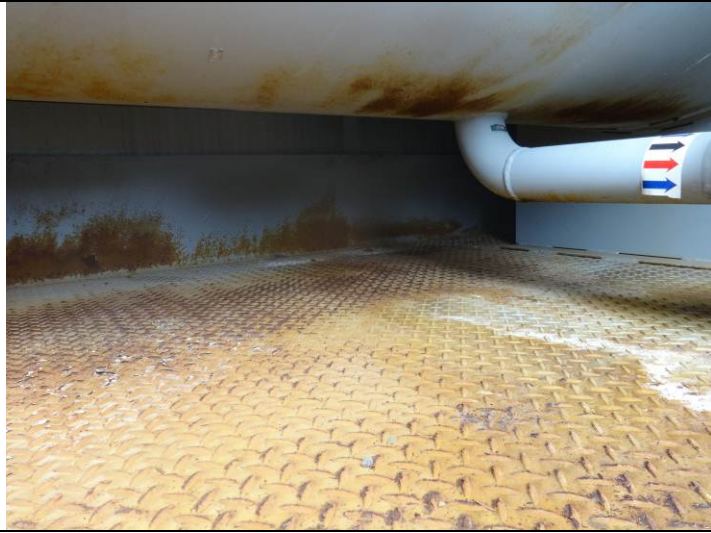
Corrosion bottom shell
