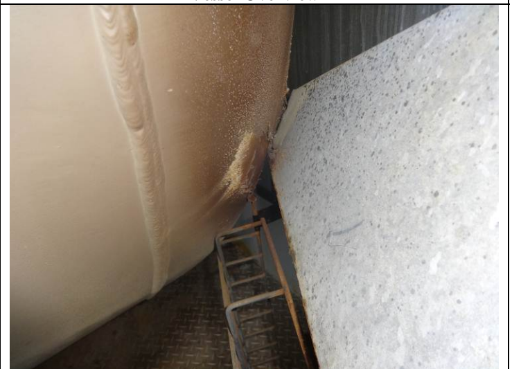
Heat damage to paint on east facing head
