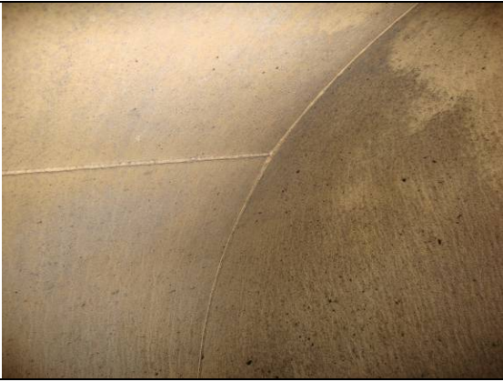
Shell coated tee weld
