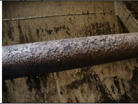
Coating blistered on heat medium piping
