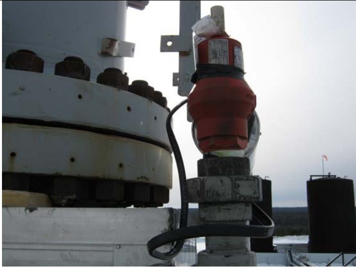
Ladder Support bent – bolts missing
