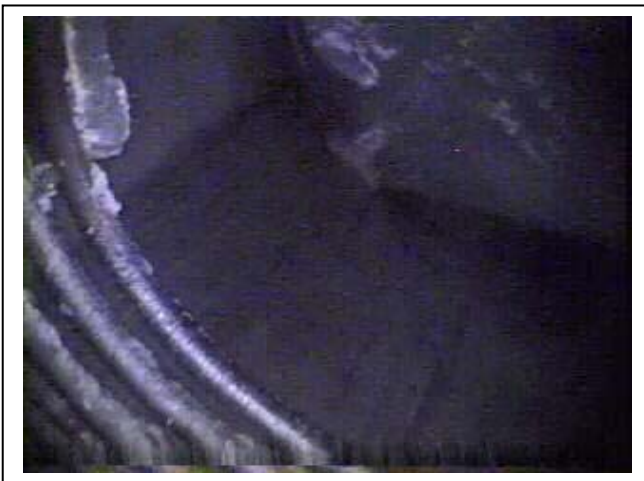
Inlet diffuser and coil in lower shell.
