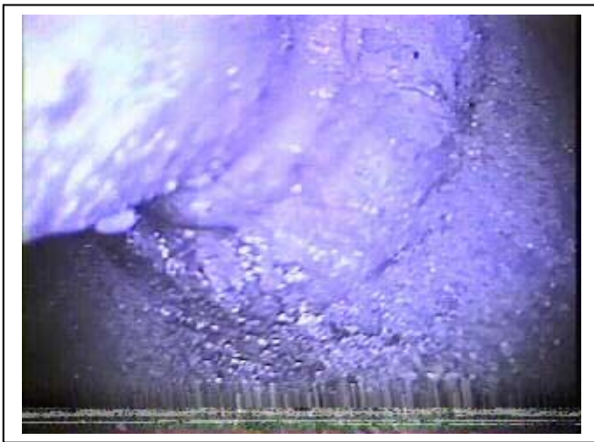
Glycol nozzle – lower shell
