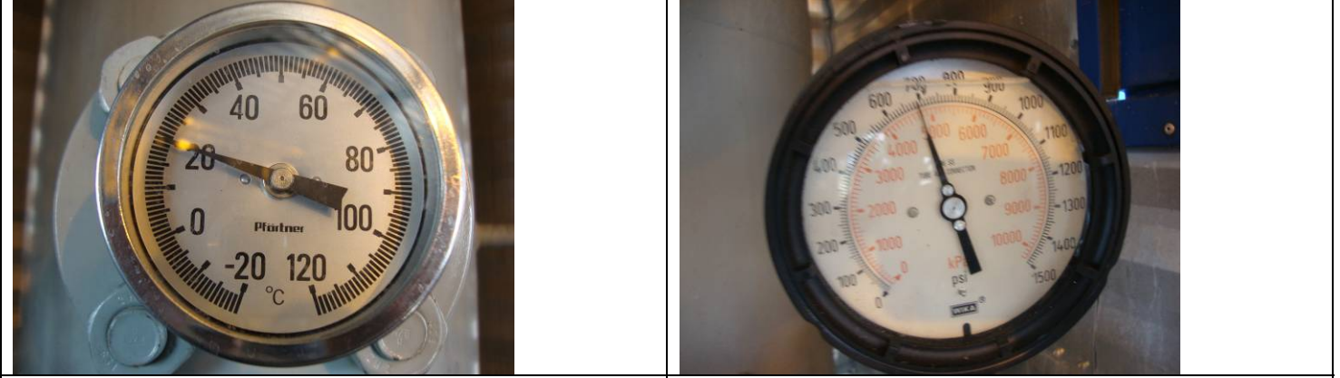
Vessel temperature gauge
