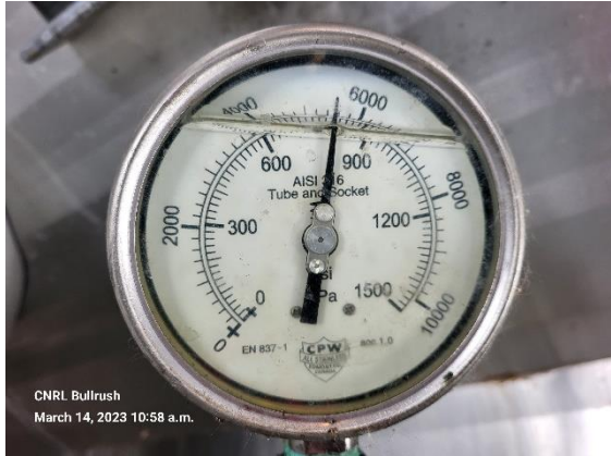
Pressure gauge overview
