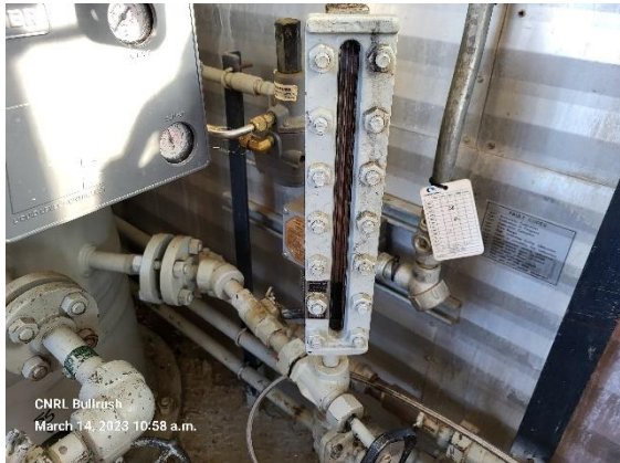
Liquid level gauge overview
