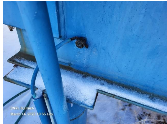
Ground cable overview
