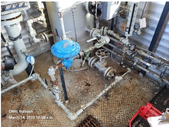
Drain piping overview
