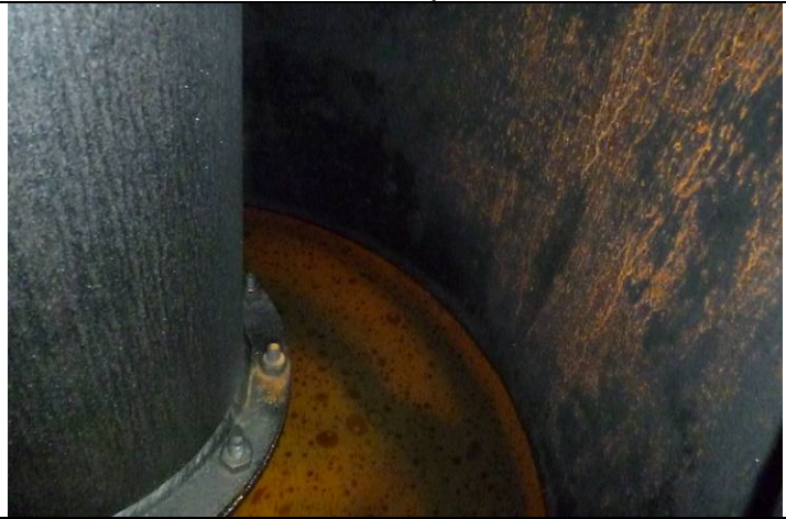
Water at bottom chimney
