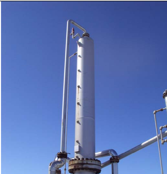
03-VESSEL OVERVIEW OUTSIDE
