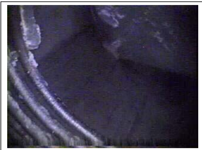
Inlet diffuser and coil in lower shell.
