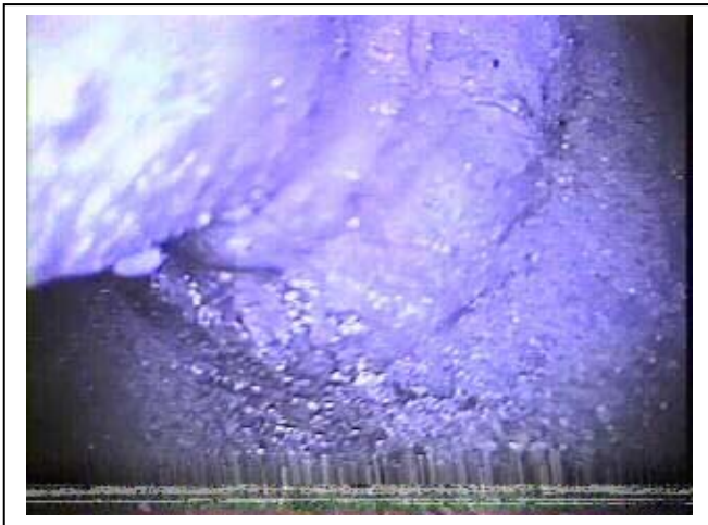
Glycol nozzle – lower shell
