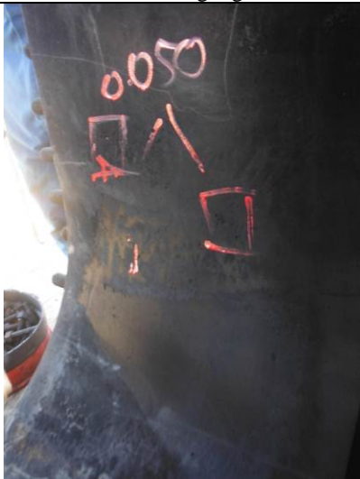
Firetube throat – corrosion to 0.050 depth
