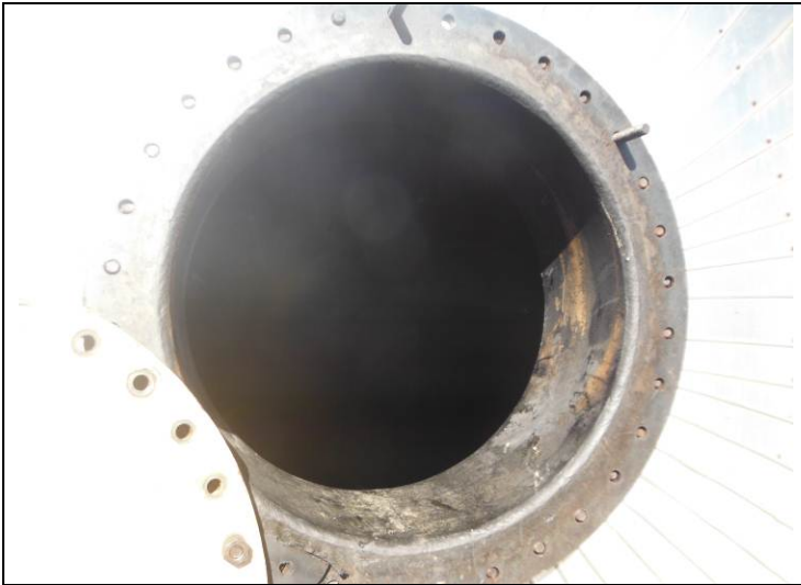
Dry side: Manway
