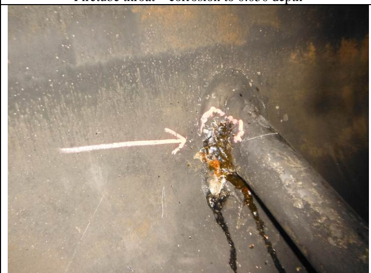
Firetube support – weld through-wall location
