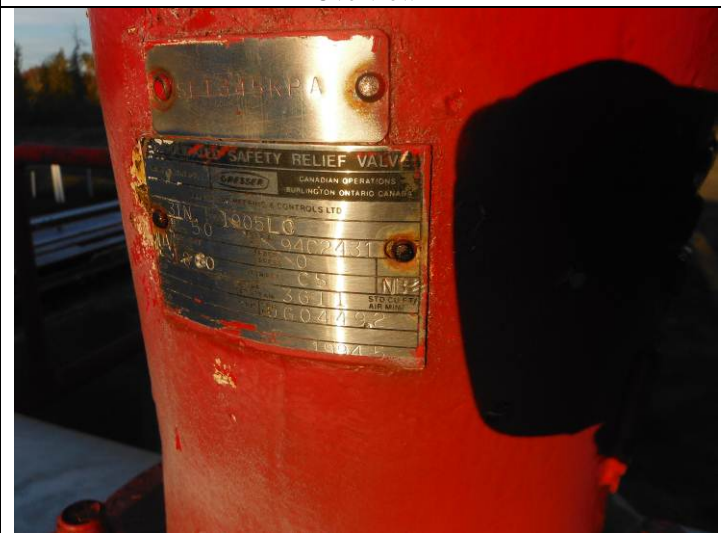
PSV data plate – service tag removed
