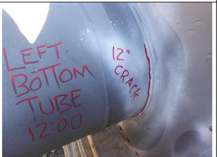
Overview Firetube LT crack location – reference MT report
