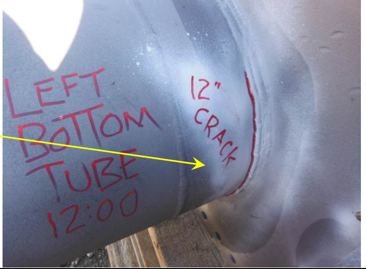
Firetube LT – 12 inch crack location
