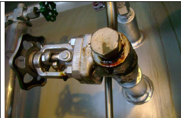
leak at valve
