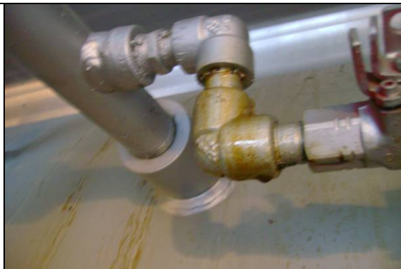
pipe threads leaking
