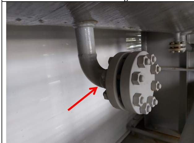
2 in 160 – 3.5/7.0mm isolated pit at DS weld
