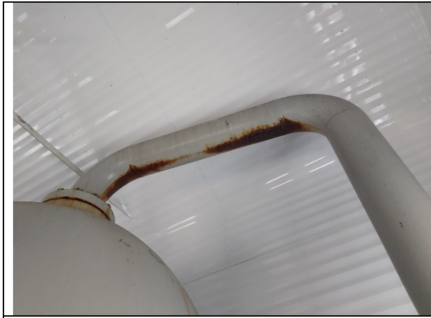
Outlet piping – surface corrosion – no pitting
