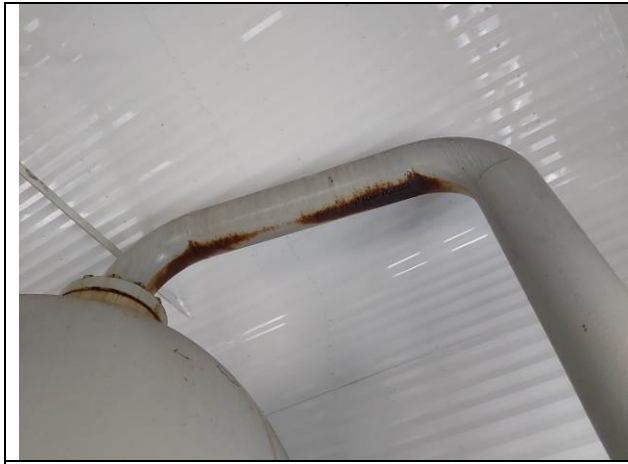
Outlet piping – surface corrosion – no pitting
