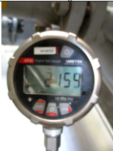
Hydro test pressure 2160 PSI
