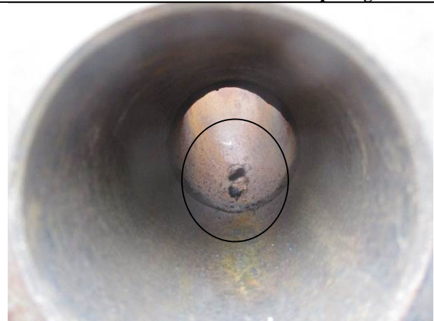
2 inch fitting – deep pitting detected on corrosion survey
