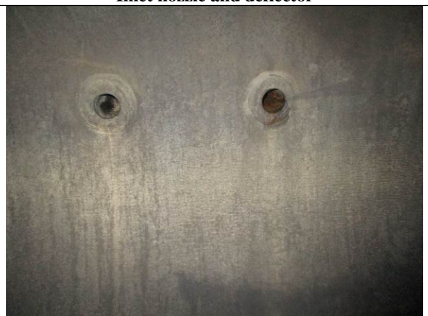
Level column nozzles
