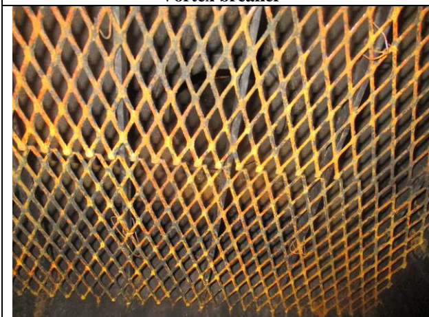
Demister screen inside cage
