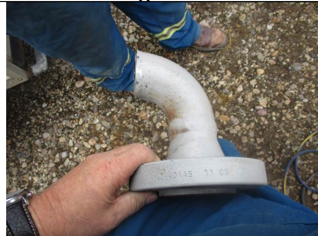
2 inch fitting cut from vessel – deep pitting detected on corrosion survey
