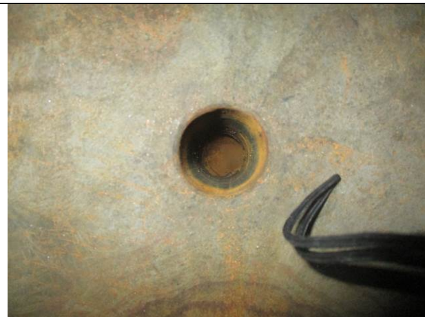
2 inch nozzle scheduled for fitting replacement
