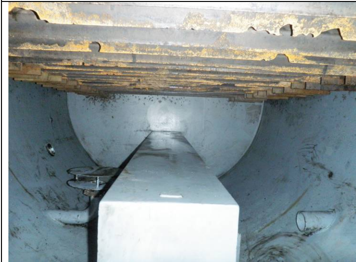
Overview (erosion on electroplating – no longer in service)
