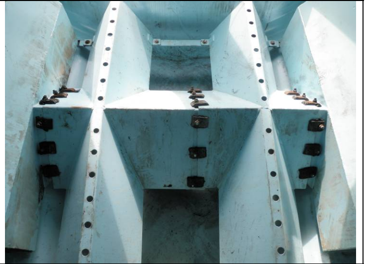
Support Structure – fire tubes
