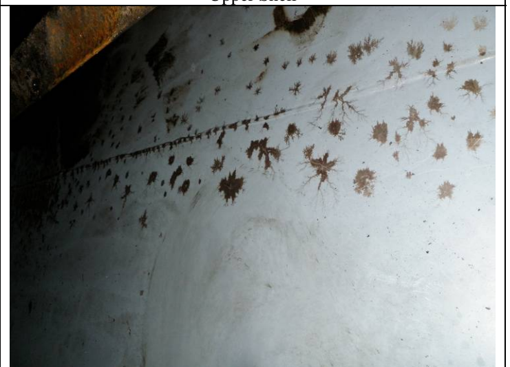
Bio-fouling on weir – surface only
