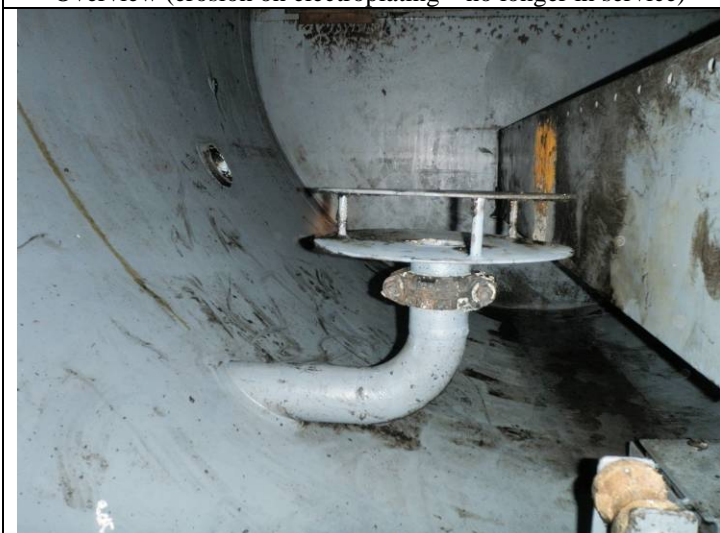
Water Dump piping
